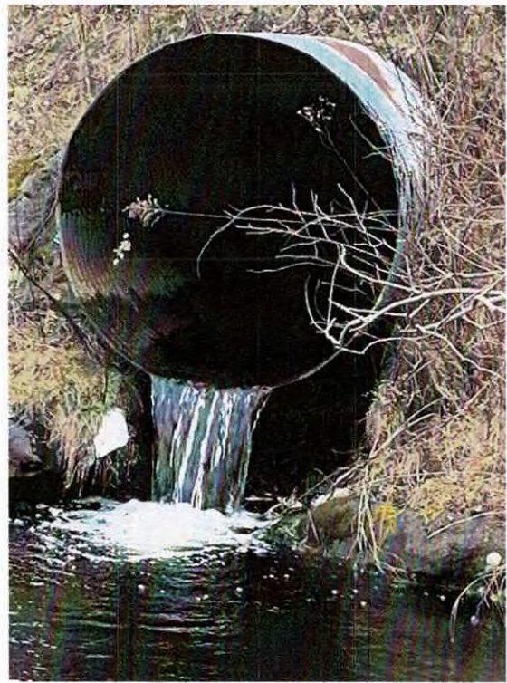
3 Feet of vertical drop to scour pool
