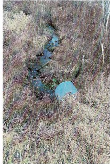
Debris interfering with flow
