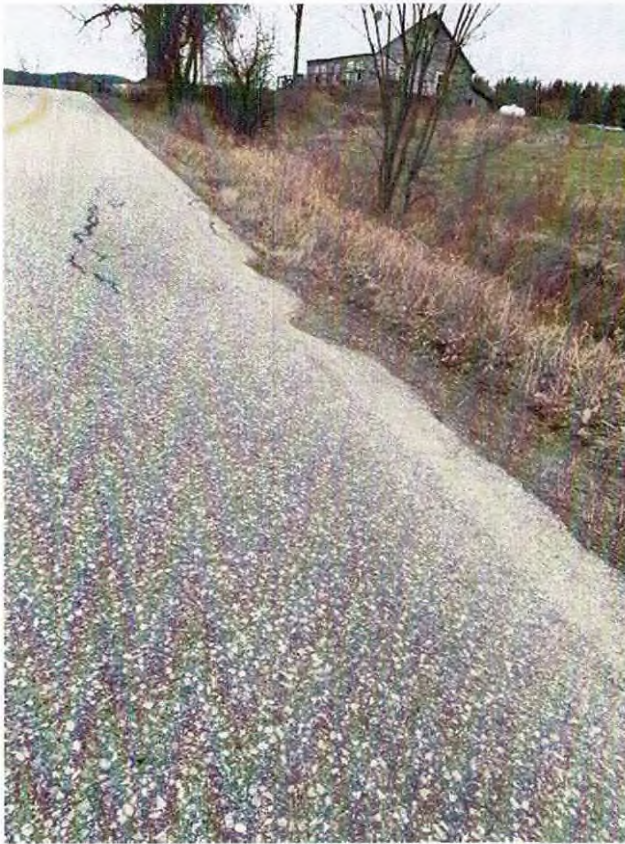
Road settling on inlet side
