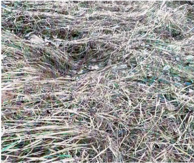
Holes developing on inlet side of shoulder
