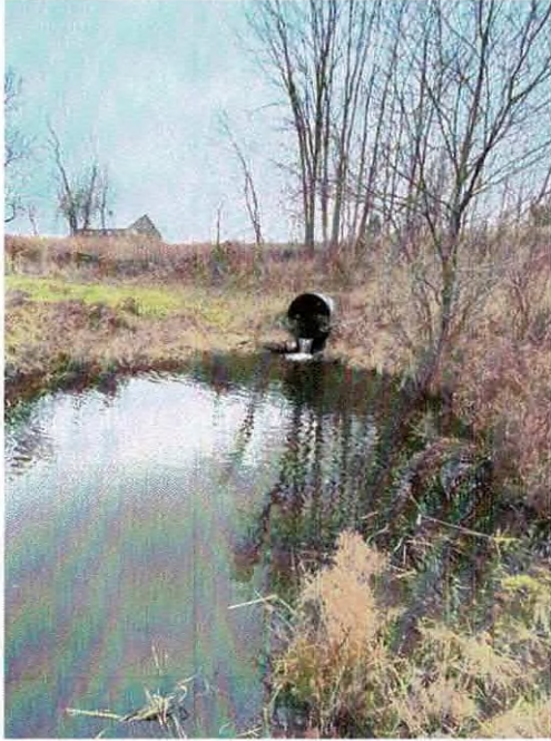
Large scour pool
